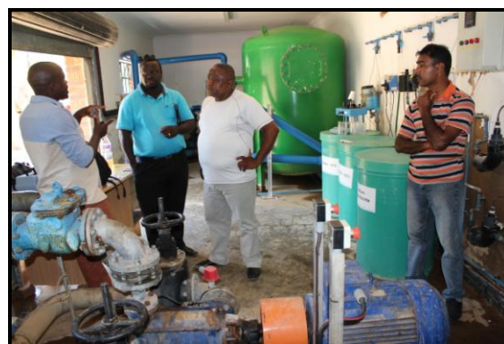
Site visit in a pumpstation by Ugu Deputy Mayor and Water Services personnel
